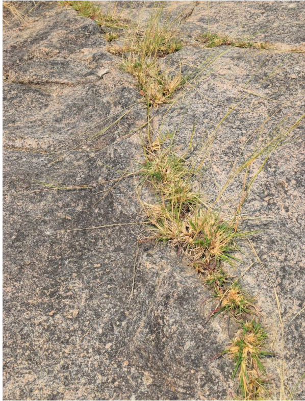
Grass growing inside the fissures on the rock
