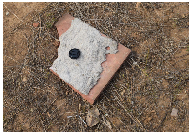
Dislodged artificial rock used for pavement
